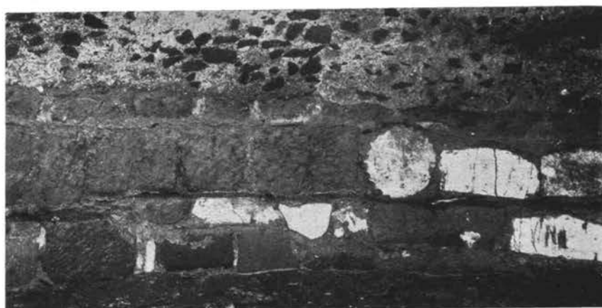
Fig. 153 — S. Lorenzo in Lucina. Foundations of inner lining wall of the apse (Photo: Sansaini).
